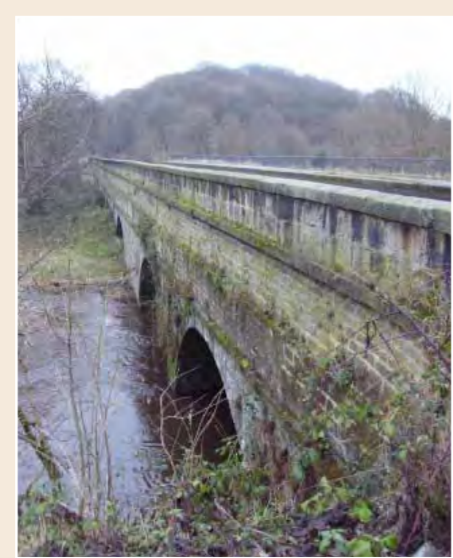
C The Seven Arches Aqueduct (Dowley Gap) was engineered by John Longbotham to the plan of James Brindley. It was built c.1773 with James Rhodes of Shipley as contractor. The Grade II Listed Building, which features voussoired segmental arches, carries the Leeds & Liverpool Canal 30ft over the River Aire. (Adapted from www.bradford.gov.uk )
